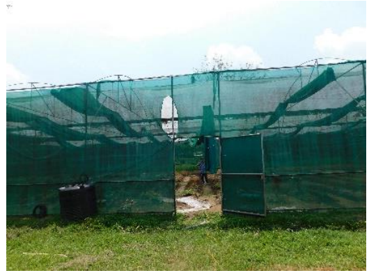
Leather Leaf Fern Polyhouse damaged by storm
