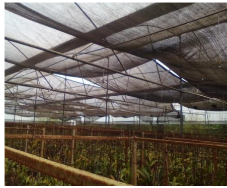
Dirty poly sheets need to be replaced
