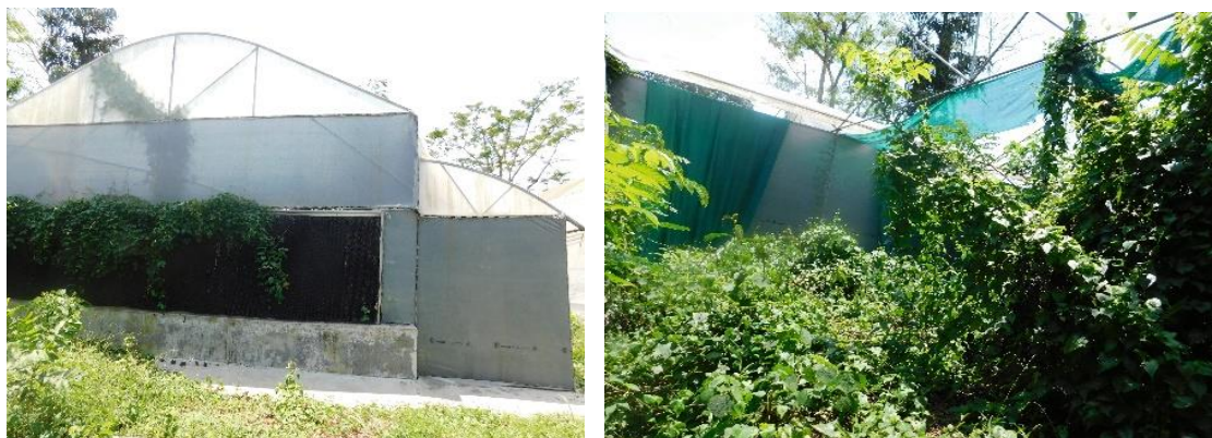
Outer & Inner view of Mist Chamber destroyed by storm
