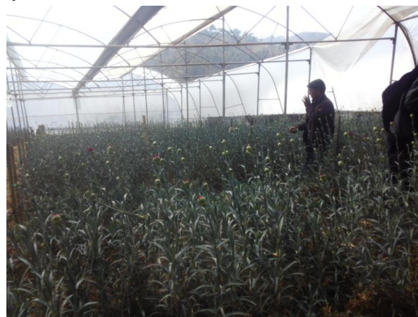
Roof of a polyhouse damaged by strong winds
