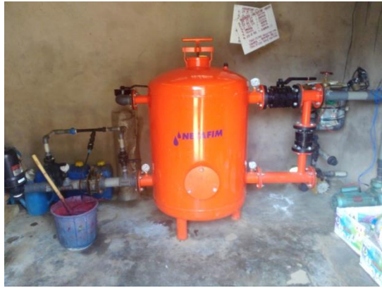
Ventury Fertigation Tank
