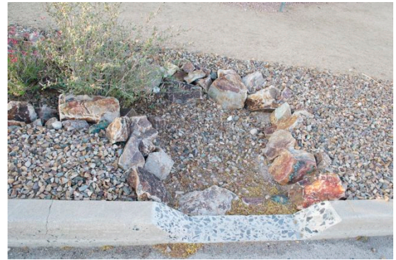
Fig. 49 Curb cut to allow water to flow in
