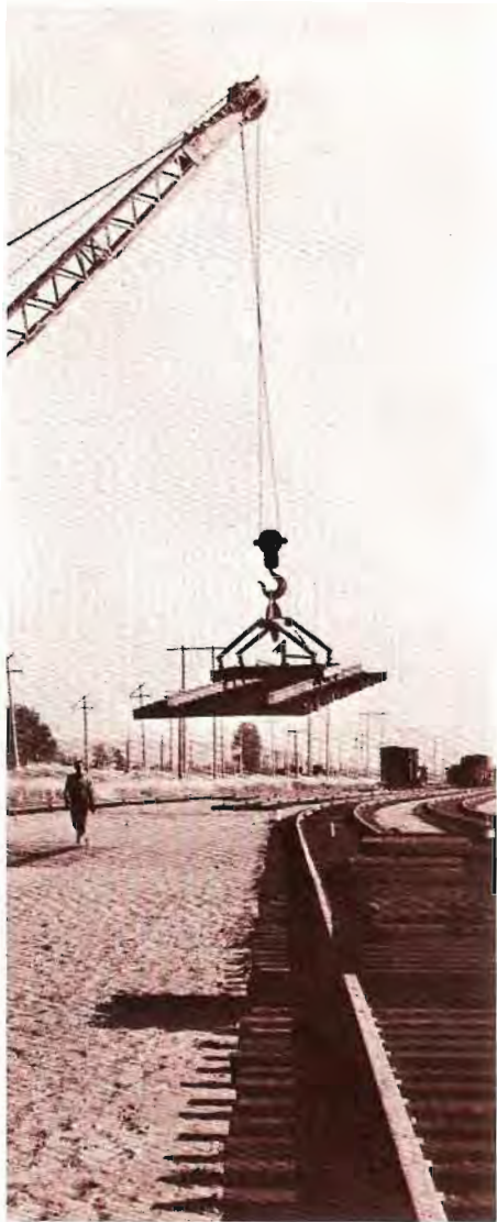
Pre-assembled 39-foot sections of track are shown being placed by a crane at the Kent, Wash., automobile marshaling complex.
