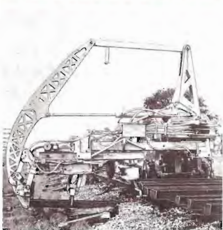
The tie injector machine shown below is the main unit of a high production gang. Average production varies between 700 and 900 ties per shift, depending on actual on-track time.
