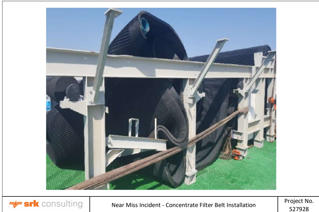
Figure 5.3: Near Miss Incident - Concentrate Filter Belt Installation
