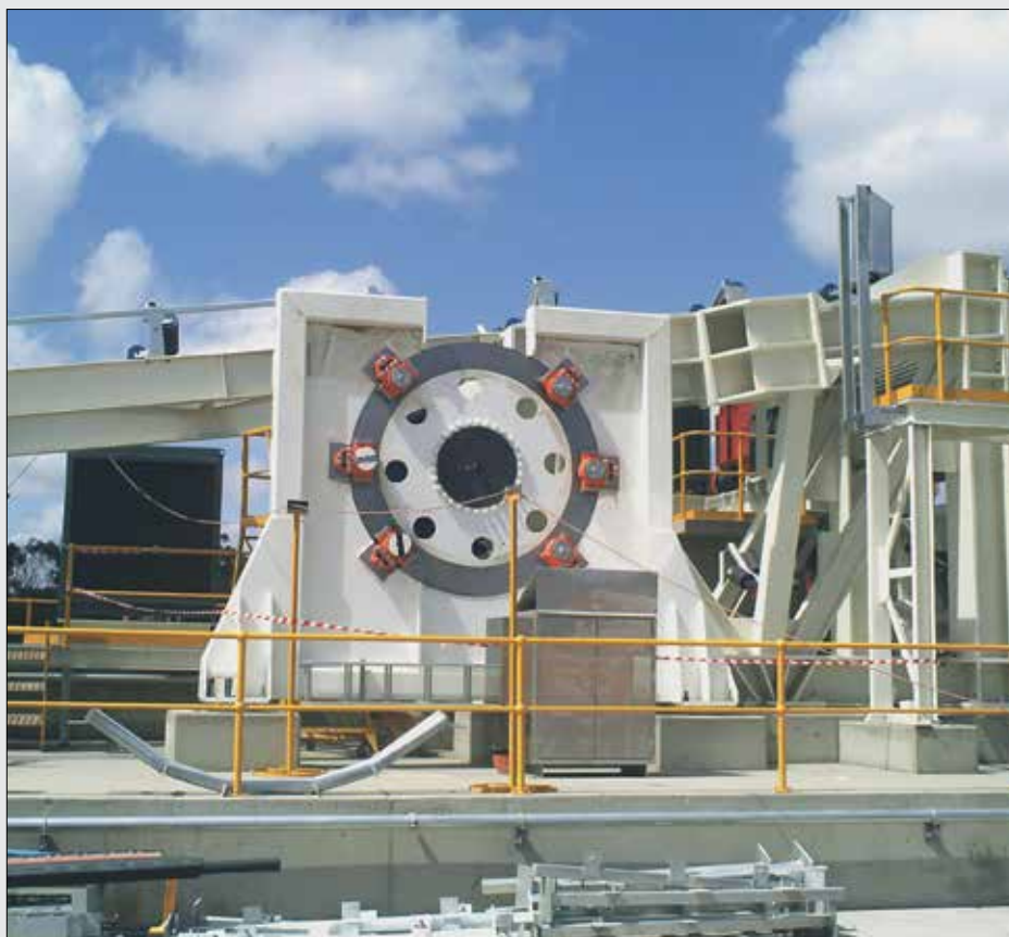
Custom Fluidpower-supplied winding equipment.
