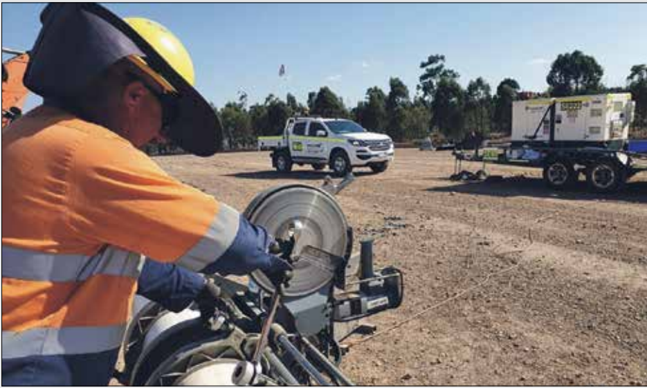
Scope Equipment Hire offers a full range of pump, pipeline and water management services.
