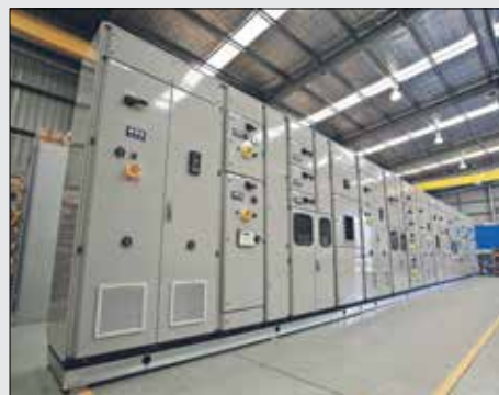
An electrical control system of the kind serviced by I S Systems.
