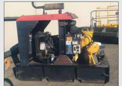
A new frame was fabricated, the roof was modified, and a new exhaust system was installed.
