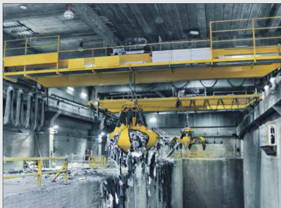
An example of a refuse crane.
