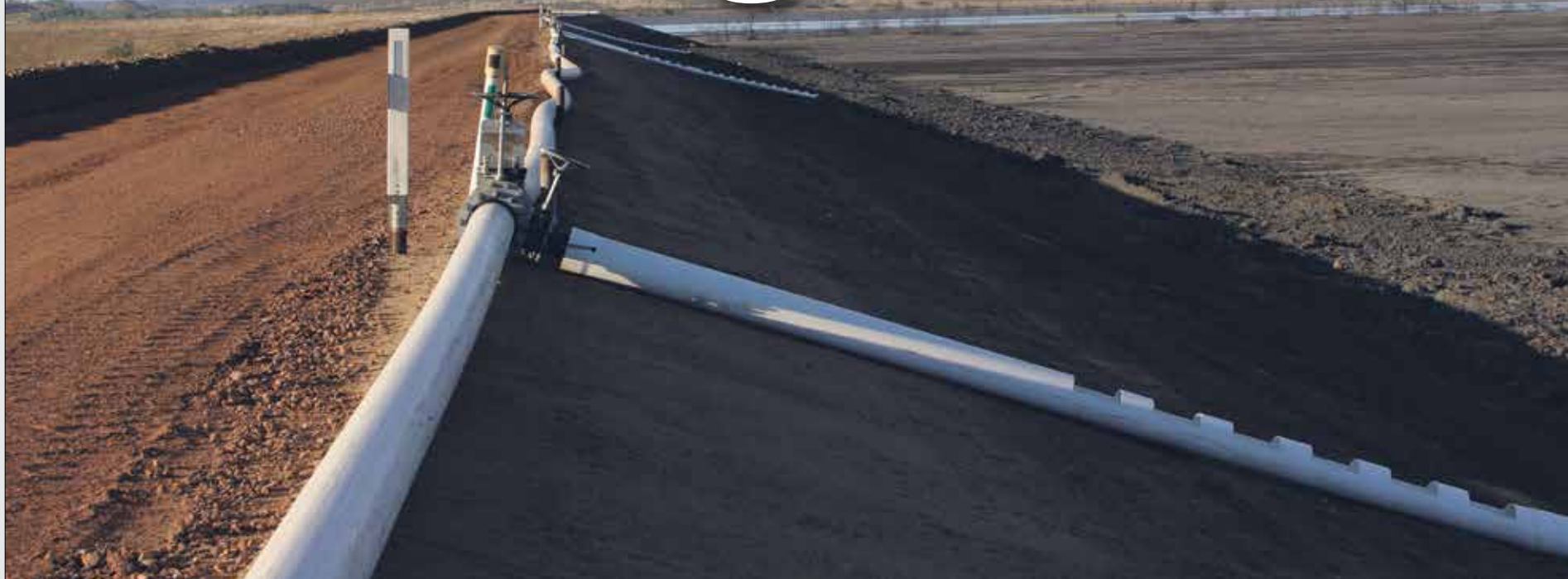
CPH specialises in mining civil works, including road, dam and levee construction, bulk earthworks, top-soil management and environmental rehabilitation.
