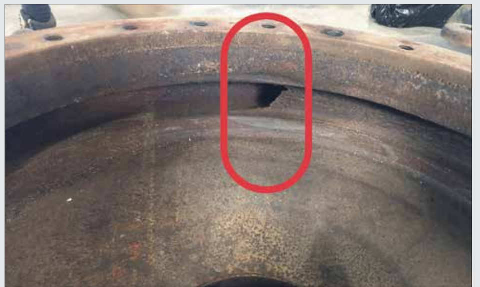
A cut water before repairs by Scope .
