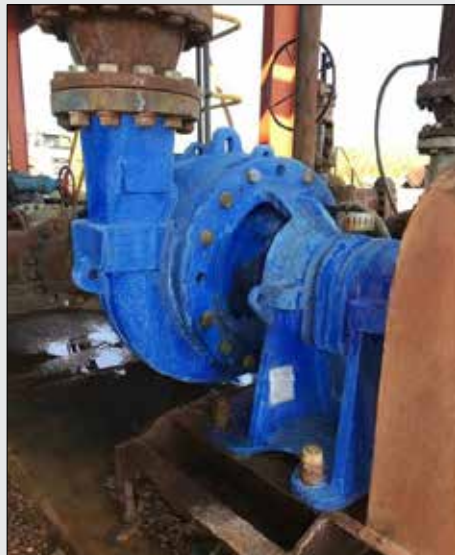
A Warman DWU pump installed on site.
