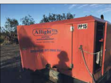
Scope took a cabinet pump destined for the scrap heap.
