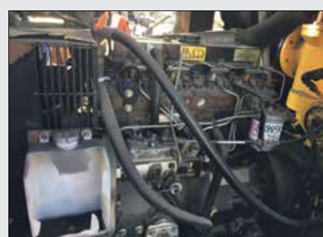
The rusted cabinet was removed.
