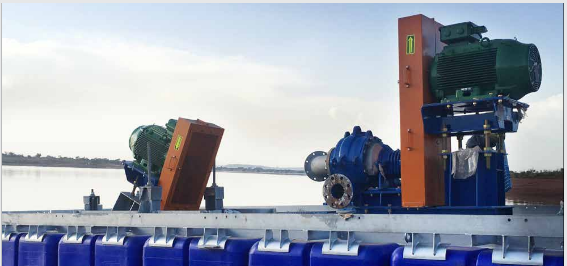
A Pontoon-mounted Warman DWU pump on site.
