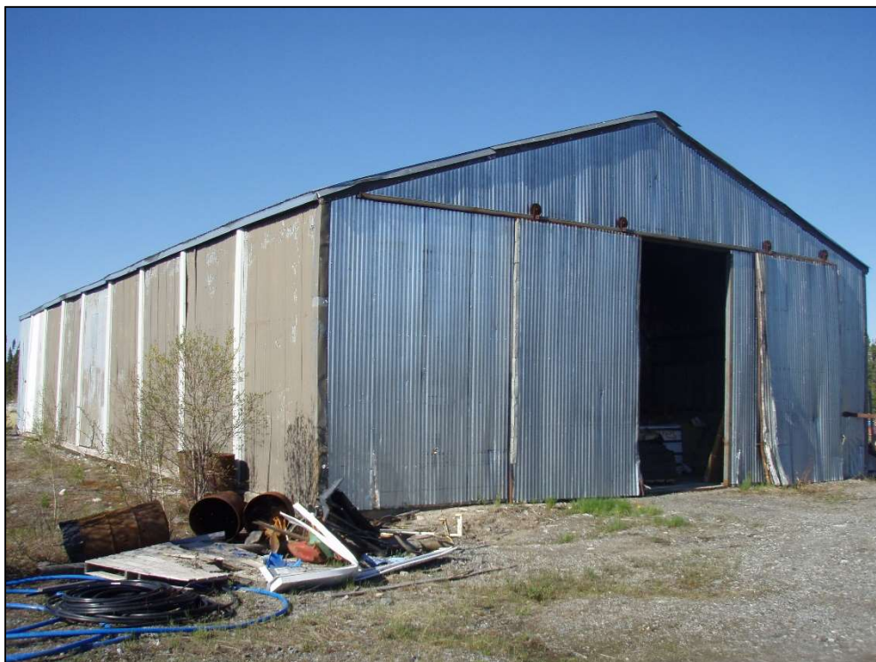
Figure 5.3 – Old garage used during the 2004 mining operations (photo taken during May 2016 site visit).
