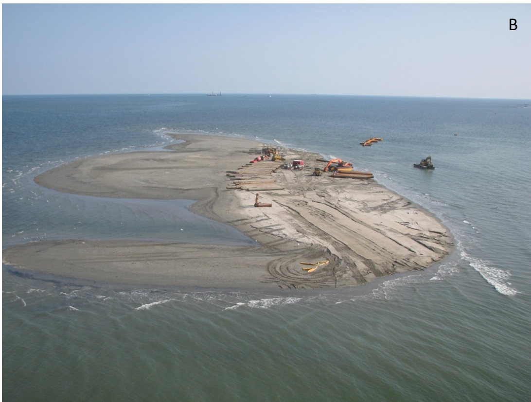
Figure 13. View of berm after several weeks of construction A. Berm in 19 July 2010. Note Dredge site at the top of the photo where sand was being sourced from Hewes Point. B. Crew is preparing to begin pumping sand after a small storm.
