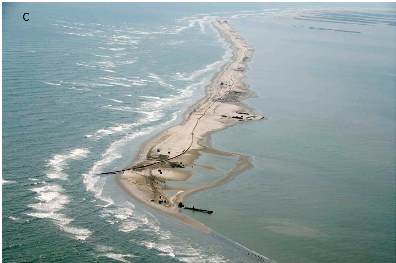
Figure 14. Photos of berm during different of construction. A. View looking north along entire length of berm north of where berm attached to the beach. B. View of middle section of the berm C. Photo of northernmost section of the berm on 3 Sept 2010 looking south.
