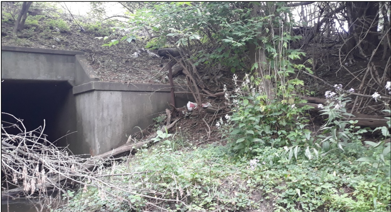
Figure 13. The many culverts throughout the project area are highly disturbed and weedy.
