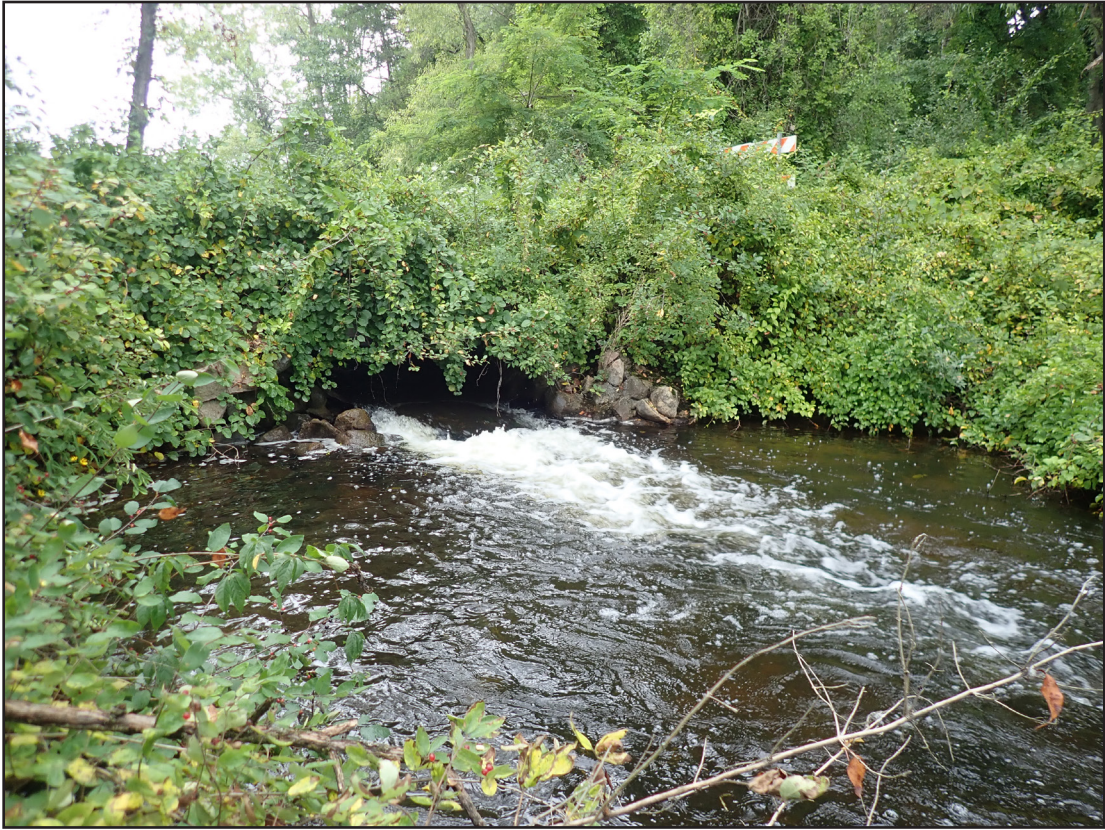
Photo 11. The downstream side of the culvert and stream crossing, looking upstream from waypoint 7.
