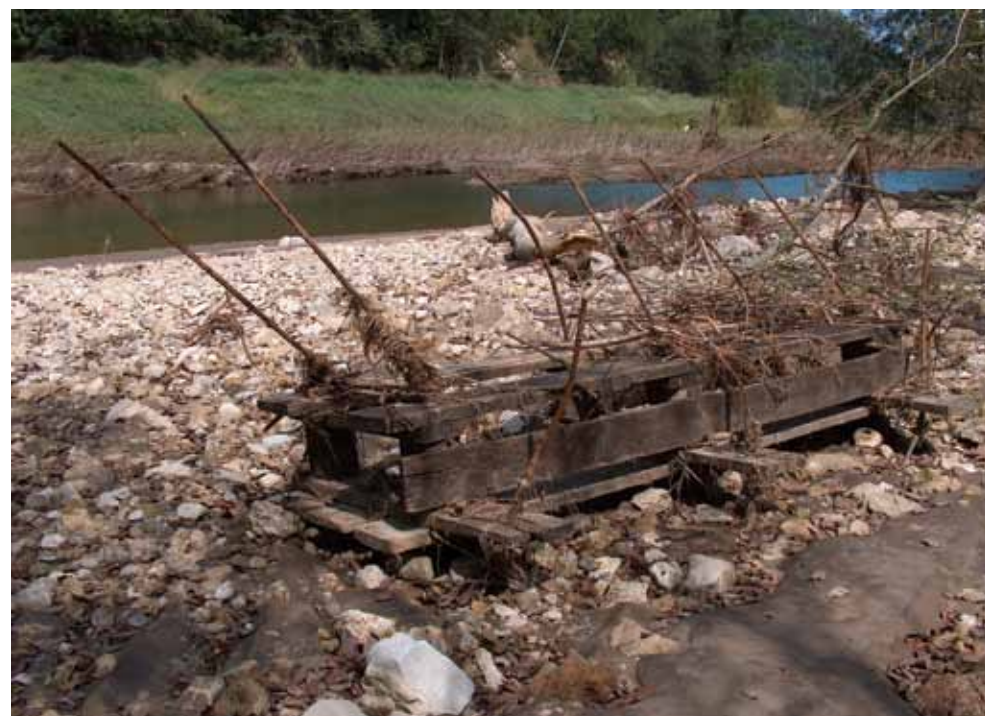
MANY HABITAT IMPROVEMENT STRUCTURES IN GARVIN BROOK, INCLUDING THIS STRUCTURE, WERE DESTROYED BY FLOODING DURING AUGUST 2007.
