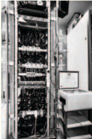
--- Public address control system, Gare Lille Flandres
