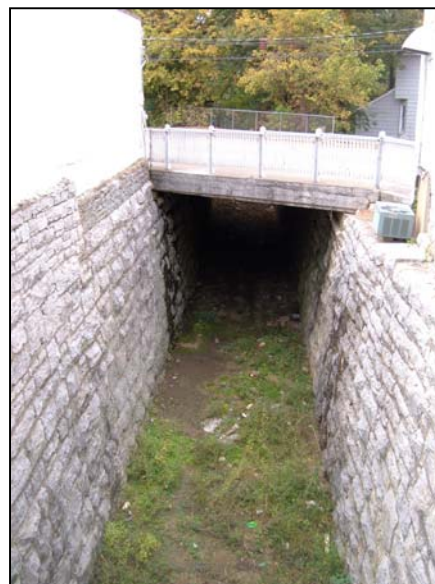
The cut stone overpass for the abandoned railroad in the 300 block of N. Main Street.
