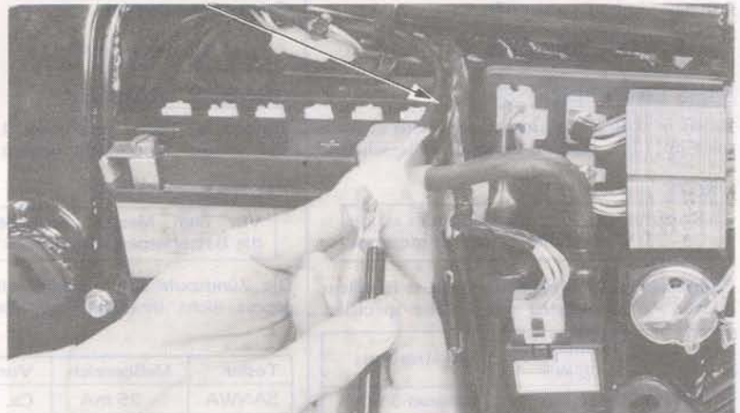
(1) PULSE GENERATOR WIRE
