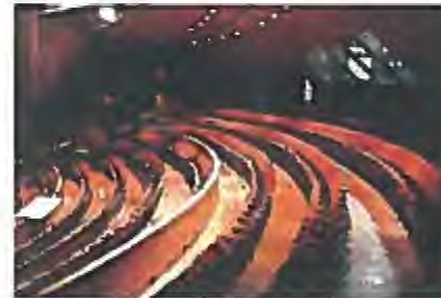
Fire sprinklers in Fain Auditorium
