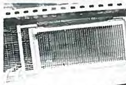
Return air systems are cross-connected in Bolin Hall
