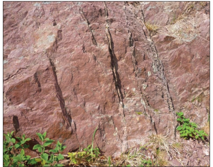
▲ Figure 3. Locality 1 - Old Red Sandstone. Typical red mudstones of the ORS with steeply inclined joints. Pale green reduction spots are possibly due to the presence of plant material in the original sediment. This would have caused the necessary chemical reducing conditions.
