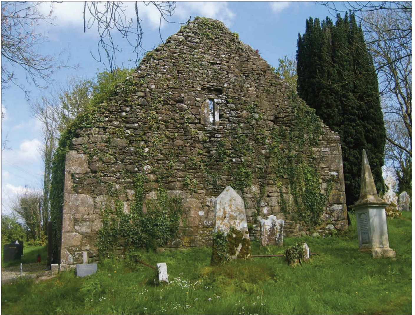
Plate VI Two phases of building can be clearly seen on this gable at the western end of the church ruins, at Kilbonane. The larger blocks of stone make up the lower courses of one phase, while smaller stones comprise the later rebuild of the church.
