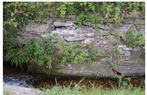
▲ PLATE XIII. The perimeter walling around Kilnaglory church and graveyard, seen from the roadside has some potentially serious patches of cracking and loss of stone.
