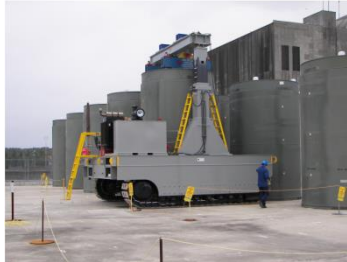
Holtec International Storage Module
