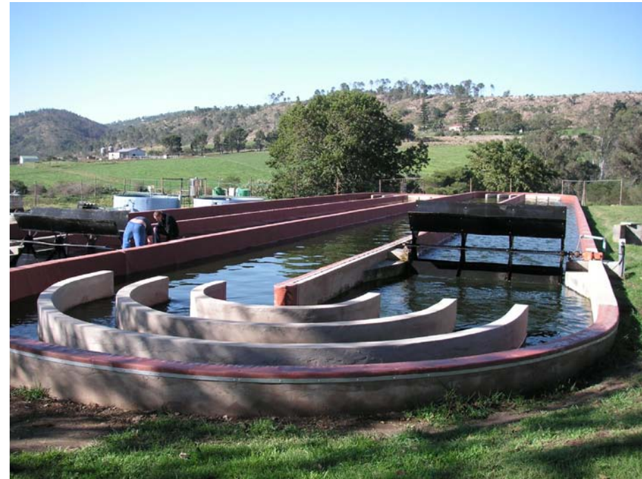
Innovative wastewater treatment at Grahamstown, South Africa (Photo courtesy of Peter Scheren)
