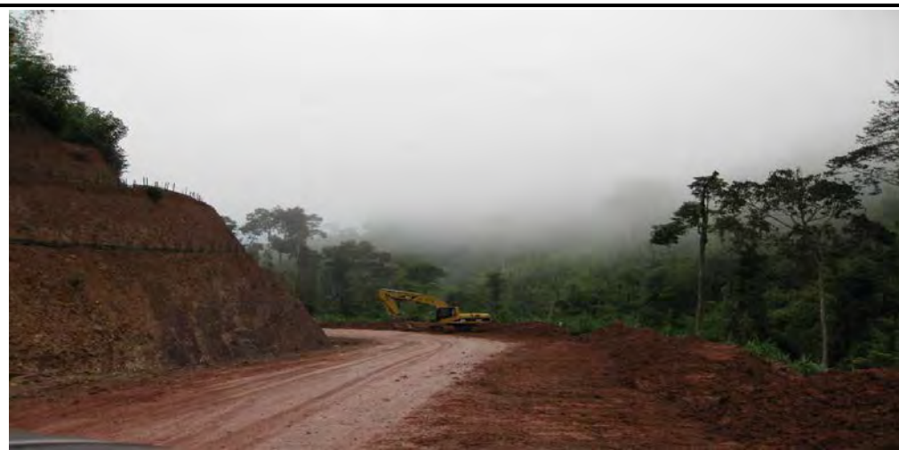
Figure 6.3 Large Sediment Load due to Unpaved Road
