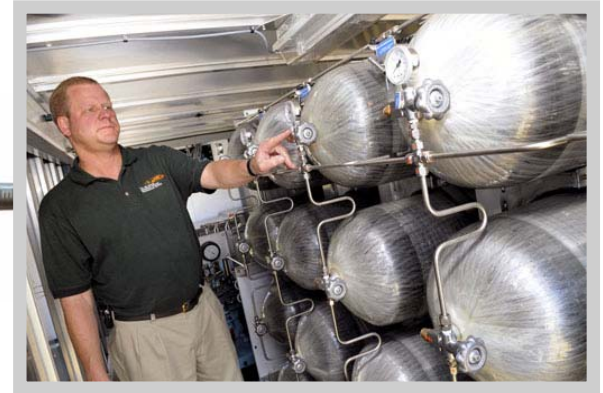
H 2 Storage Facility
