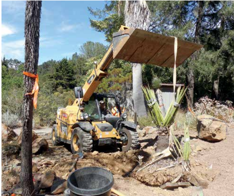
A large specimen of Mojave yucca ( Yucca schidigera ) was carefully moved as construction began on one of the Desert section’s new rock gardens.
