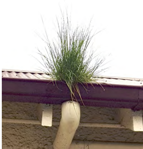
A grass valiantly poking out above the gutter.
