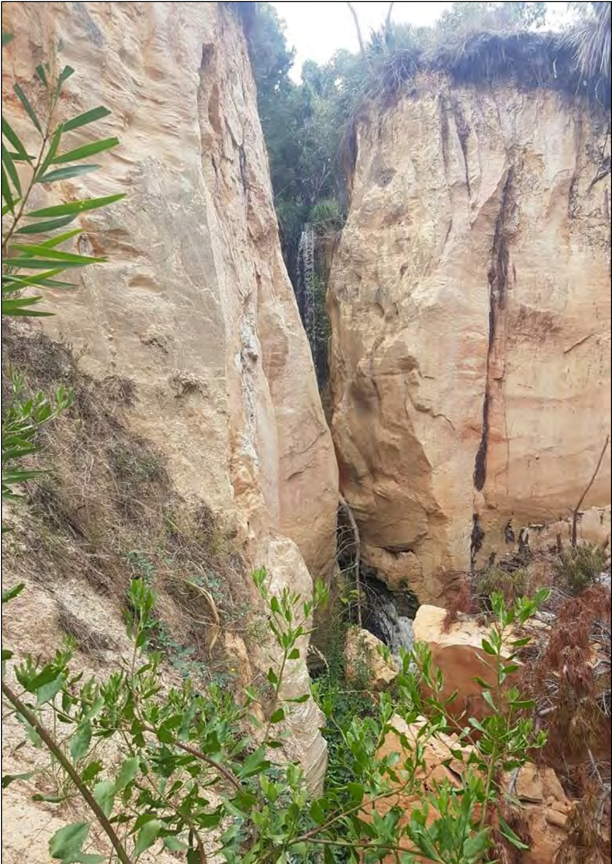
Figure 3.7: The present appearance of the artificial waterfall created at the terminus for the upslope bypass drain constructed at Nangkita in the early 1890s. Note the substantial effects of 125 years of erosion.
