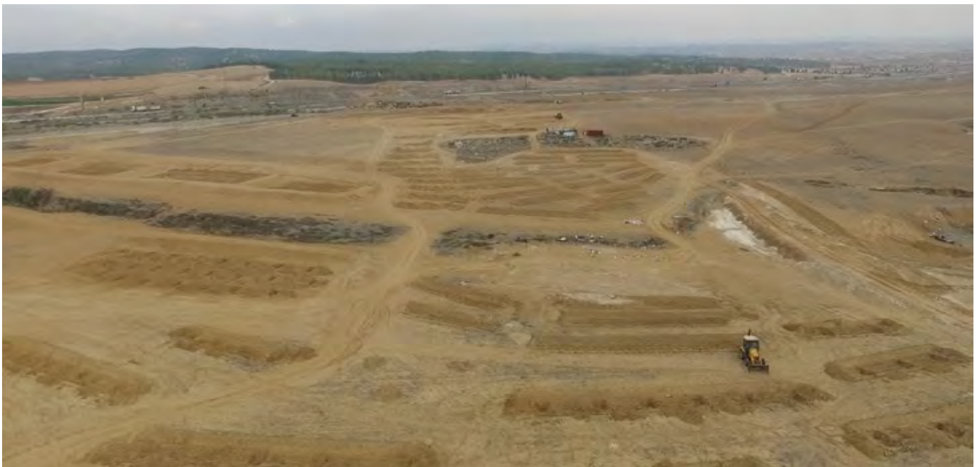
Earthworks for planting preparation in a loess area in the Northern Negev.
