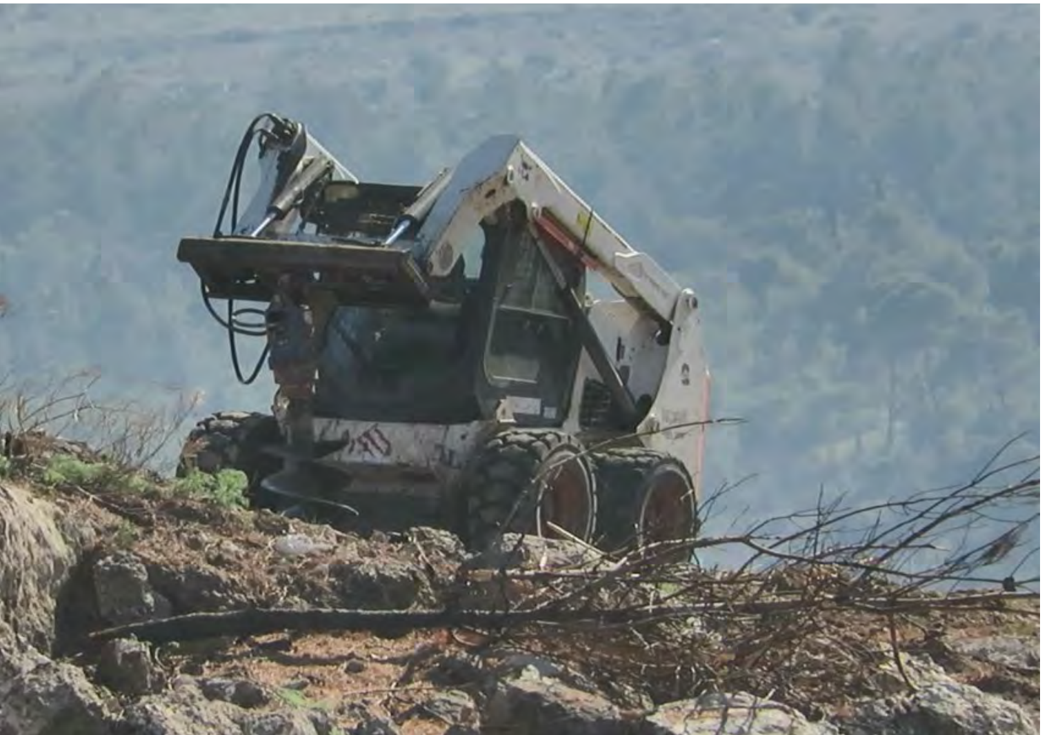
KKL tractor excavating “planting holes” in a rocky area in the Judean Lowlands. Photo: Avraham Shaked
