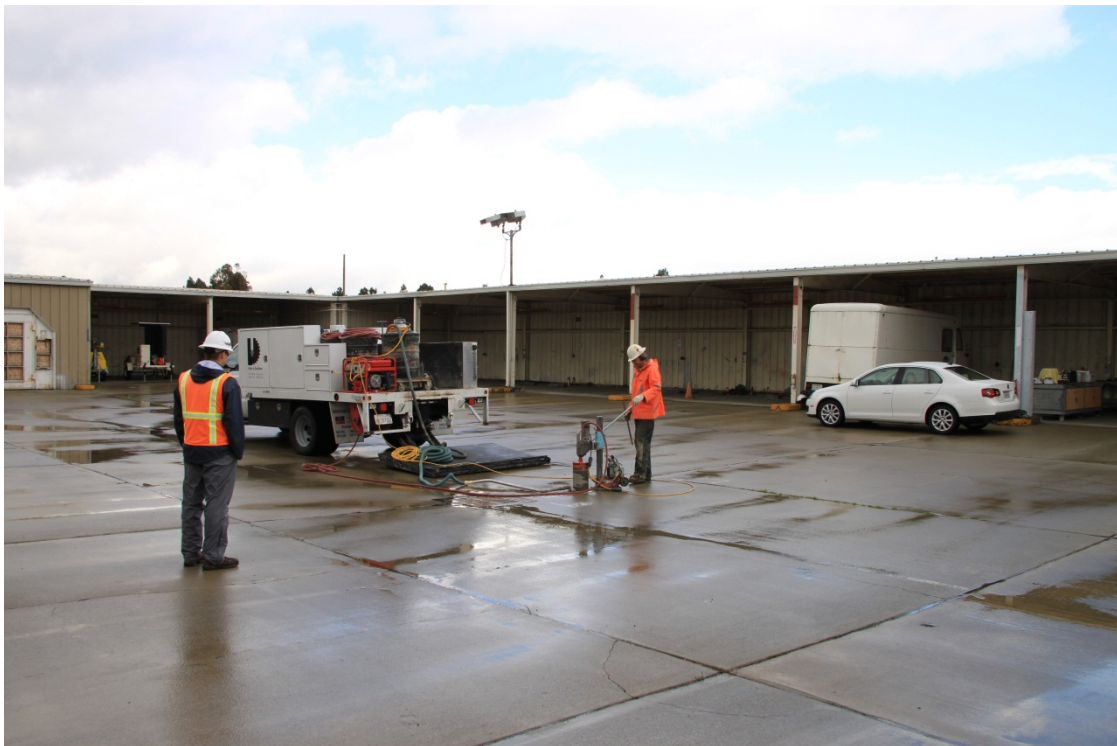
Photograph D-18. Core cutting in Bldg. 544 courtyard (note bldg. open to courtyard)
