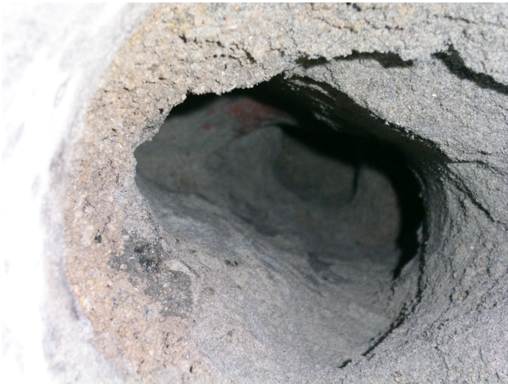
Photograph D-14. Exposed red clay pipeline (upper left)
