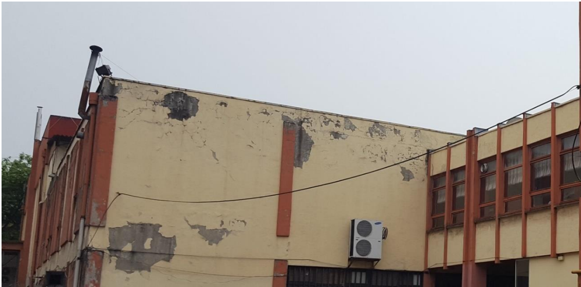
Photo 8. Damage to the facade exposed to rainwater
