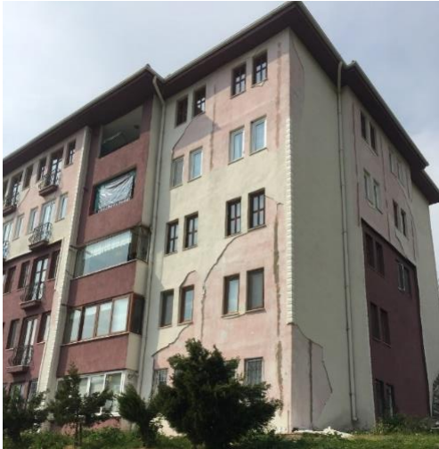
Fig. 30.. Type-2.1 facade deterioration
