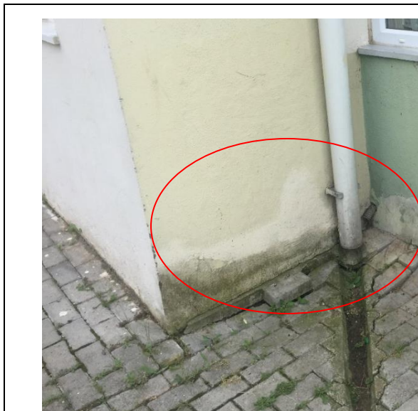
Fig.10 Type-1.2 Efflorescence (southeast)
