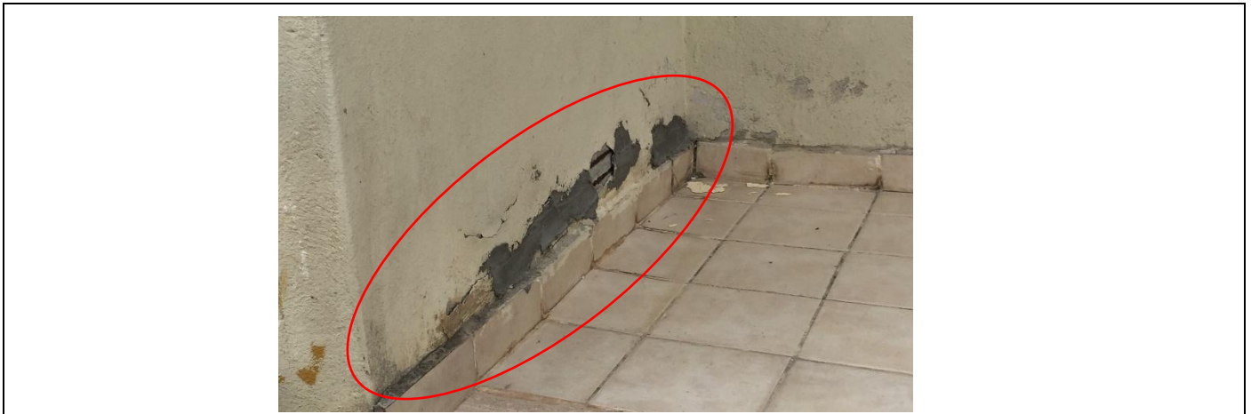
Fig. 34. Type-1.1 corrosion (northeast)
