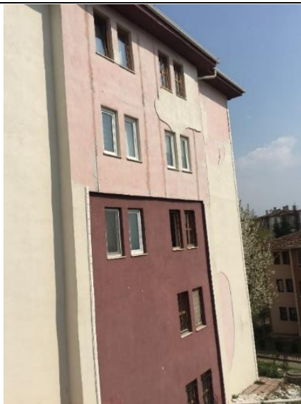
Fig.32. Type-2.1 Facade deterioration (southeast)
