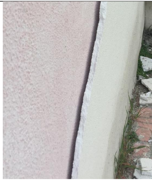
Fig 33. Type-2.1 Facade deterioration (southeast)
