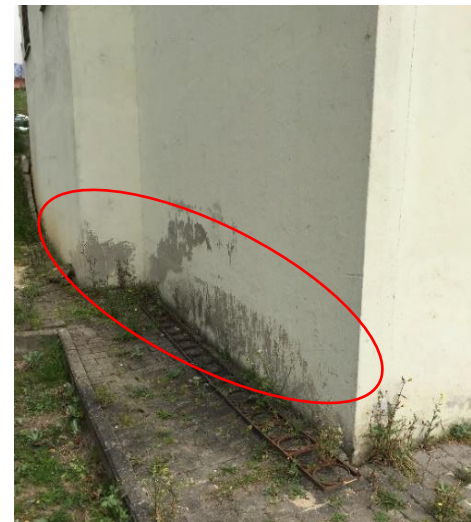
Fig.9 Type-1.1 efflorescence (northwest)
