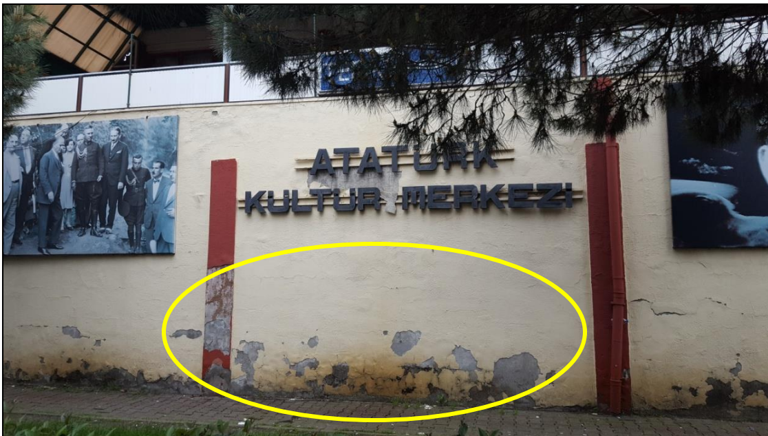
Photo 1. Damage to the facade exposed to water.
