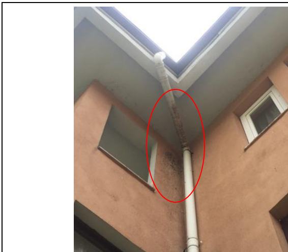
Fig.28.Type-2.2 Rain downpipe and bird droppings
