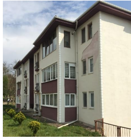
Fig. 31.. Type-2.1 facade deterioration
