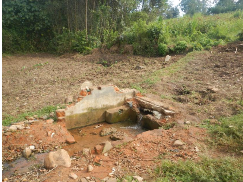
Plate 1: Dilapidated Khalala community water spring
