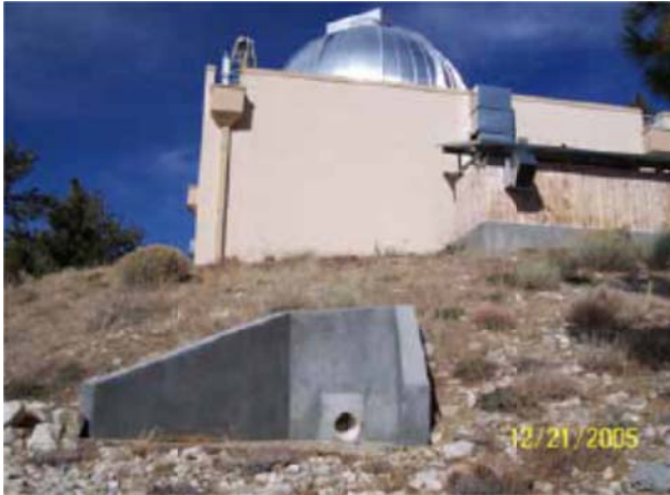
Figure 3-19. Roof Drain Conveyance System at Building TM-29
