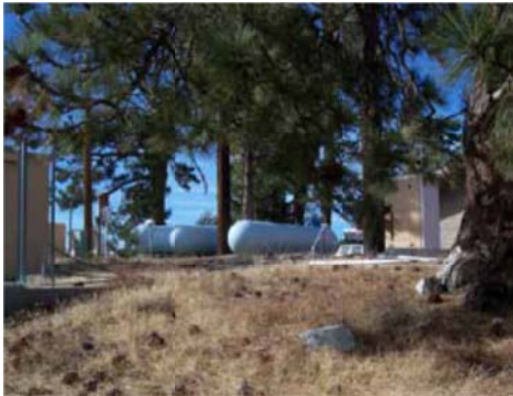
4478 Figure 3-18. Liquid Propane Tanks at TMF
