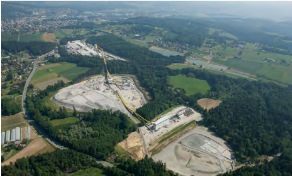
Figure 4 Site installation of lot KAT 2 at "Leibensfeld" (in the back of the picture) with storage and material treatment facilities
