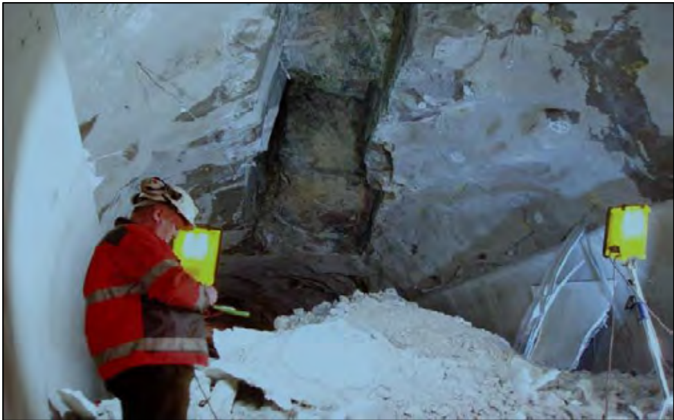
Figure 1. Photo of the collapsed area in the roof of the Hanekleiv tunnel and the material from the cave-in on the floor of the tunnel (Nilsen, 2012).
