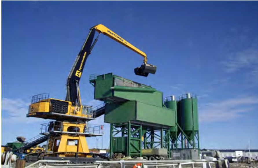
Figure 4. The process stabilisation equipment of Biomaa Ltd (Lemminkäinen)
