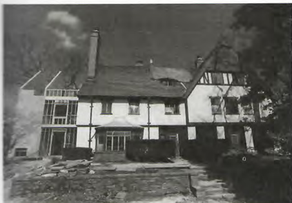
A substantial addition to Treetops's left side will allow the building to house about 50 NIMH employees.
