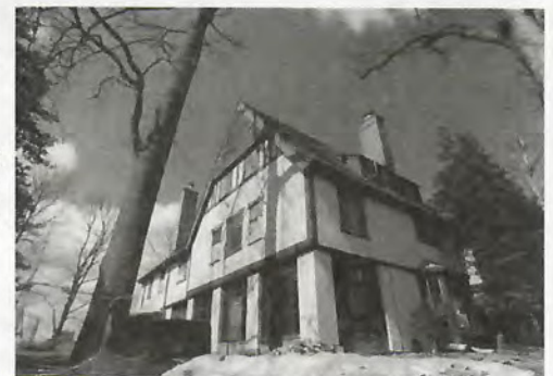
The last of "Treetops," Bldg. 15K is in the final stages of a major renovation project.
