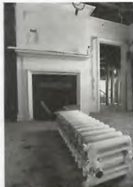
The original fireplaces will remain, but the outdated radiator heating system will not.
