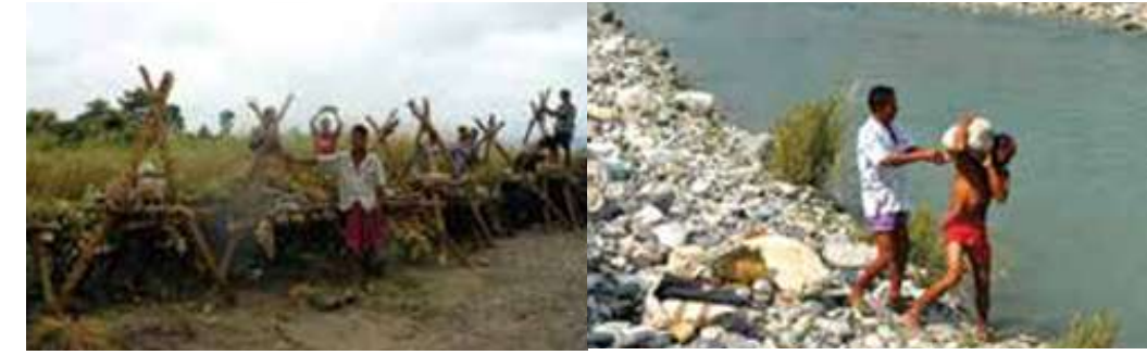
Collective labour for construction of deflectors ( porcupines ) and dong - bundhs Stream channelisation during dry season upon downstream demand
