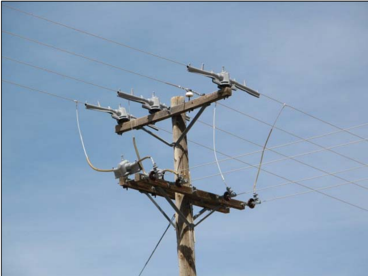
Figure 6-3. Retrofit pole with conductor wire covers and insulator covers and extenders.
