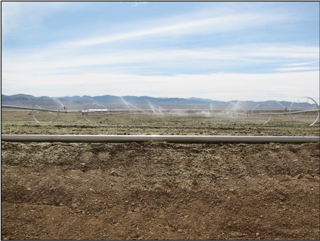
Figure 7-10. Irrigation system in operation at CAU 577 Cells 19/20. (Photo taken March 17, 2022, by D.B. Hall)
