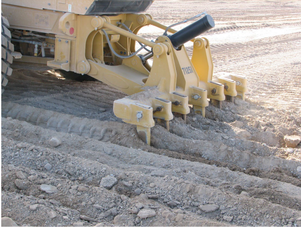
Figure 7-5. Ripping CAU 577 Cells 19/20 with road grader to alleviate soil compaction. (Photo taken March 3, 2022, by D.B. Hall)
