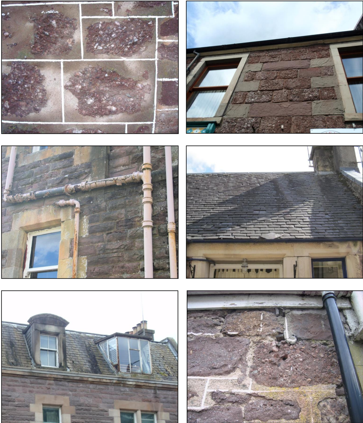
Figure 18 Examples of the most serious conservation issues affecting buildings in the CCA.
