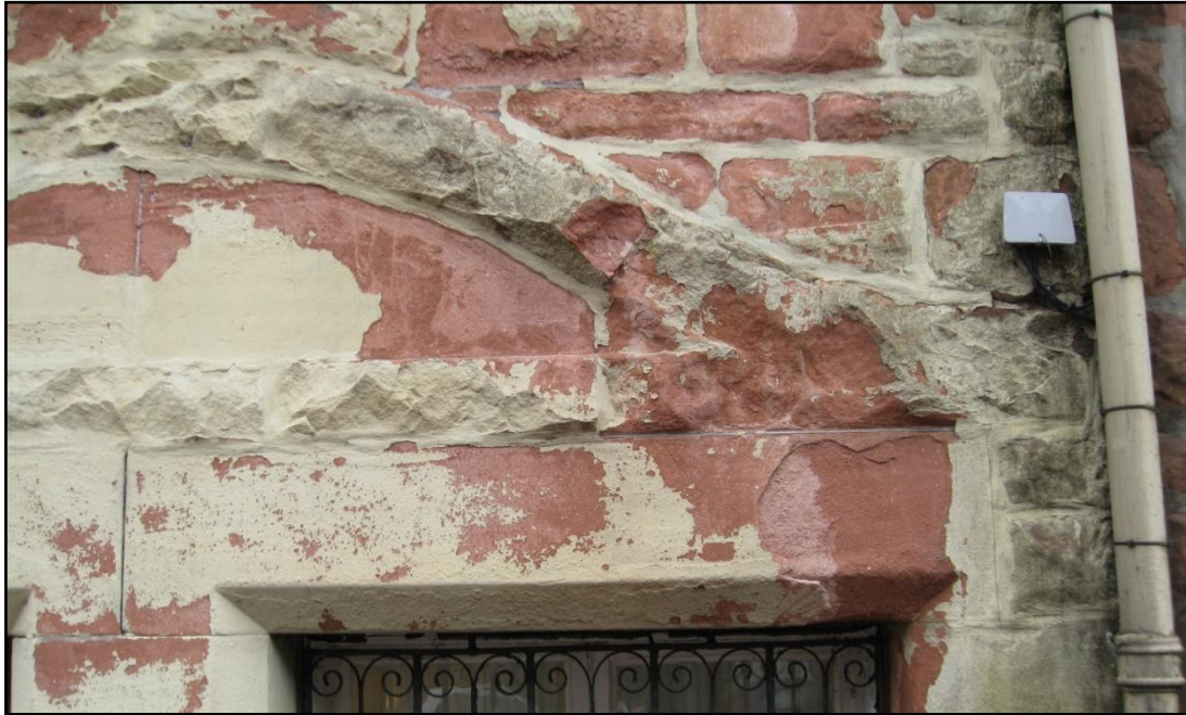
Figure 5 Damage to a hood mould on Cross Street elevation. It is possible that the complete removal of this water shedding element was thought to be a better solution than repairing and restoring the protruding masonry; however, this has only led to the enhanced decay of the stone facade below.
