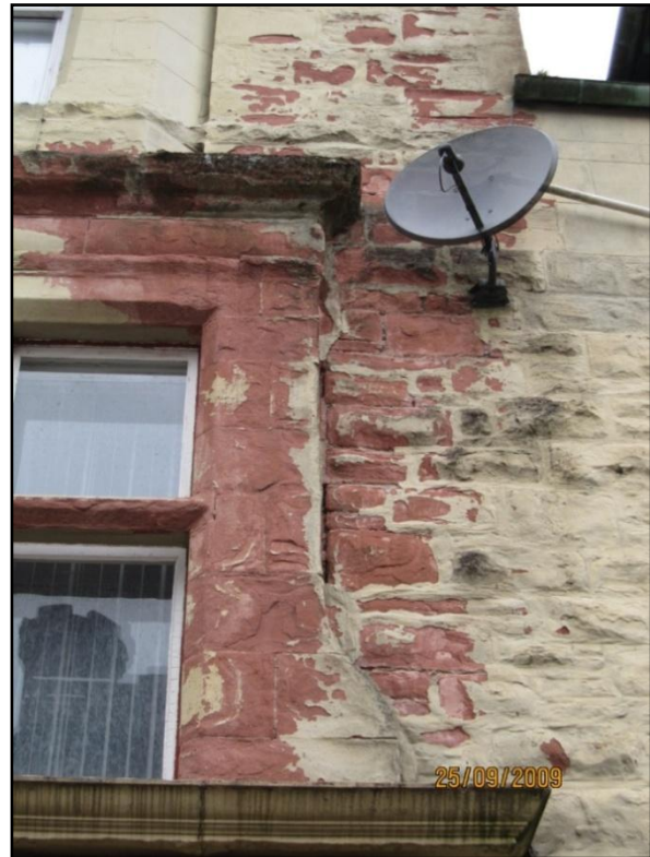
Figure 2 Cross Street elevation. Examples of scaling, crumbling and areas where repointing is required. Paintwork is flaking off.
