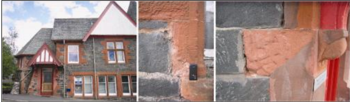
Figure 8 Main Street and Trossachs Road, Aberfoyle. C(s) listed building (c.1886) with squared and snecked whinstone rubble and red sandstone dressings. The red sandstone dressings are similar to the 'Desirables' stone type and display some of the similar features of stone decay.
