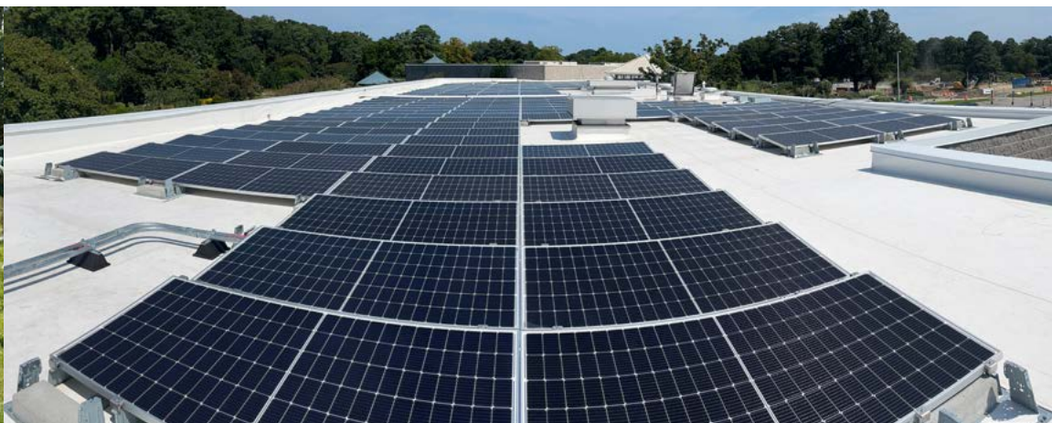
New Solar Panels Installed on the roof of Baker Hall & Education Center
