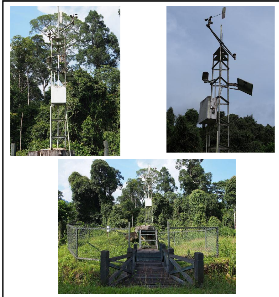
Picture 5.1: Automatic weather Station (AWS) at MBSC
