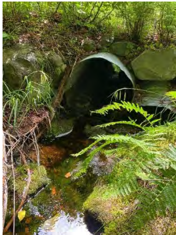
Photo 9. Evidence of alteration along WC5.
