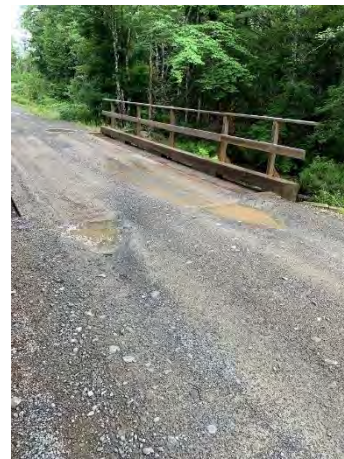
Photo 6. Evidence of alteration along WC3.
