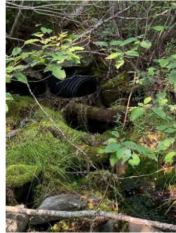
Photo 2. Evidence of alteration along WC1.
