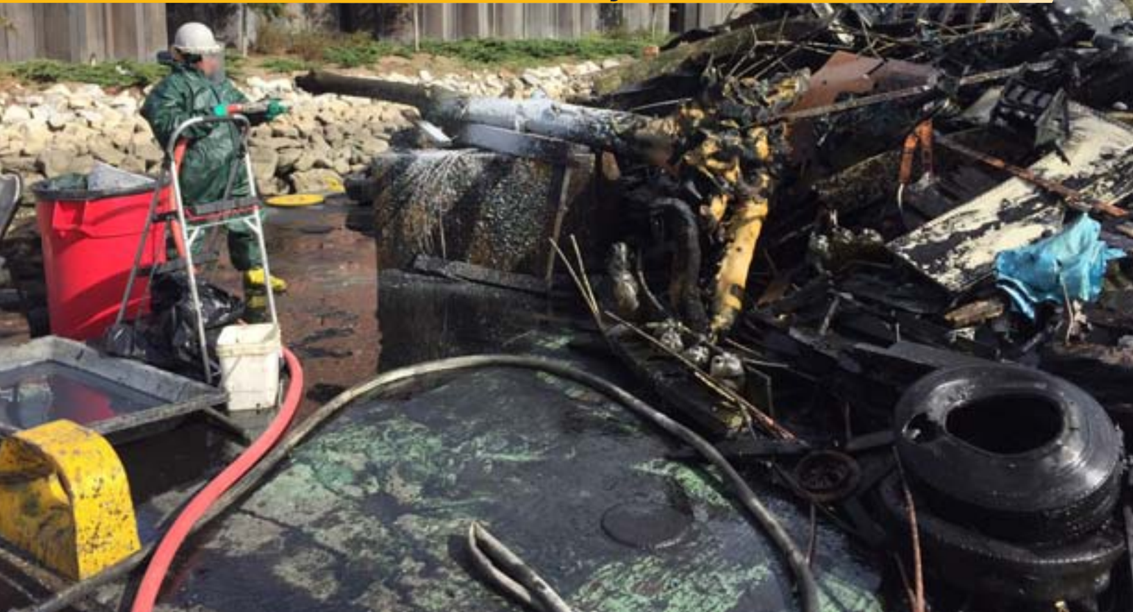
A worker prepares to wash down debris removed from the 4th Street Basin in front of the Whole Foods store. All items removed from the basin have been stockpiled at a nearby staging area and will be evaluated for archeological value before being hauled to a disposal site. Photo courtesy of USEPA.
