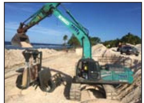
The aid project rebuilt borrow pits left from WWII, when U.S. Marines built an airstrip and Navy base, leaving huge plots of excavated land.
