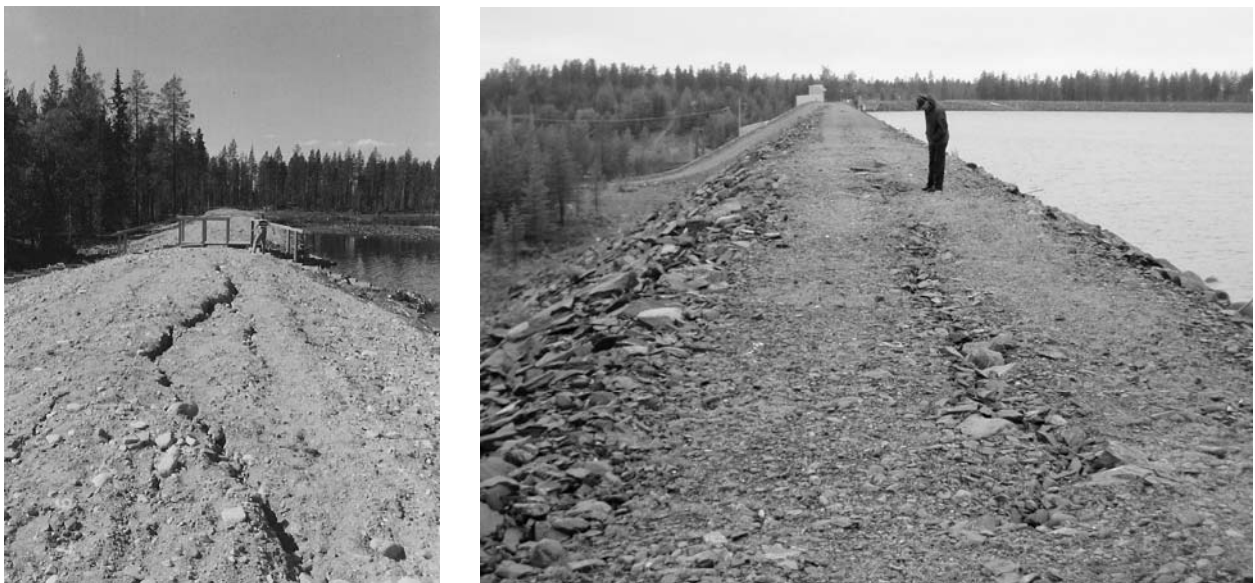
Figure 1: Longitudinal frost crack in a) a minor earth dam in Yläliesijoki in Finland, photo by A. Leskelä and b) the zoned Grytfors rock fill dam in Sweden, photo by I. Ekström.
