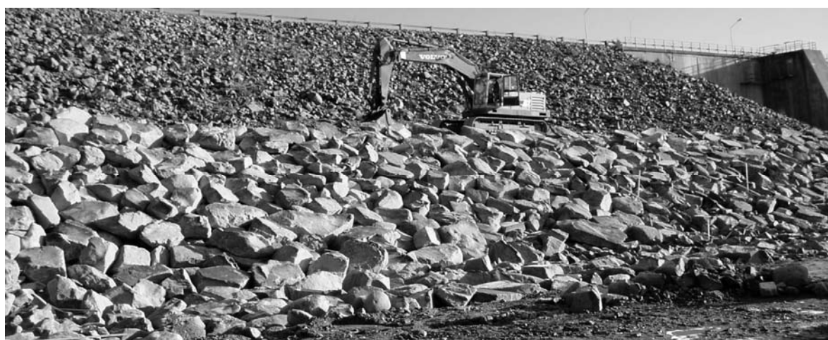
Figure 10: Construction of the berm half way up to the crest of the dam
