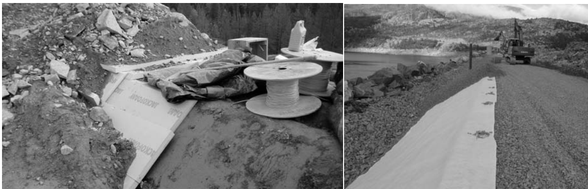
Figure 8: a) Frost protection in Grytfors dam in northern Sweden: insulation of raised moraine core, photo by I. Ekström. b) Use of light weight foam glass aggregate as the sloping insulation in the Suorva Västra dam, photo by Å. Nilsson.
