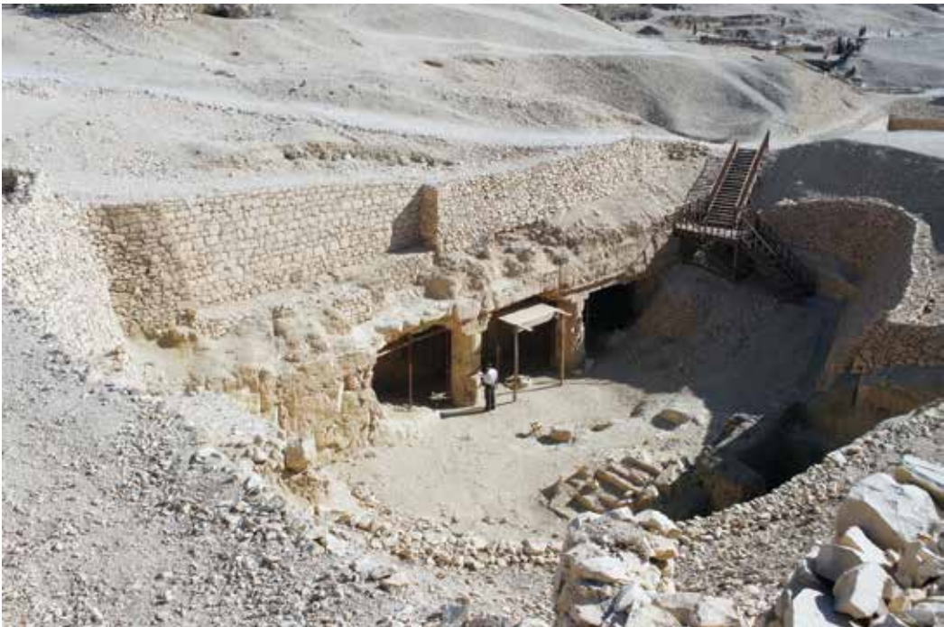
Figures 18–20. Clockwise from top left: (18) Conservation team at work on fragments of the South Well of Ramesses III, Medinet Habu; (19) Conservation team restoring blocks of the well housing, South Well of Ramesses III, Medinet Habu; (20) View of the court, Tomb of Nefsekheru (TT 107) (photos: Ray Johnson)
