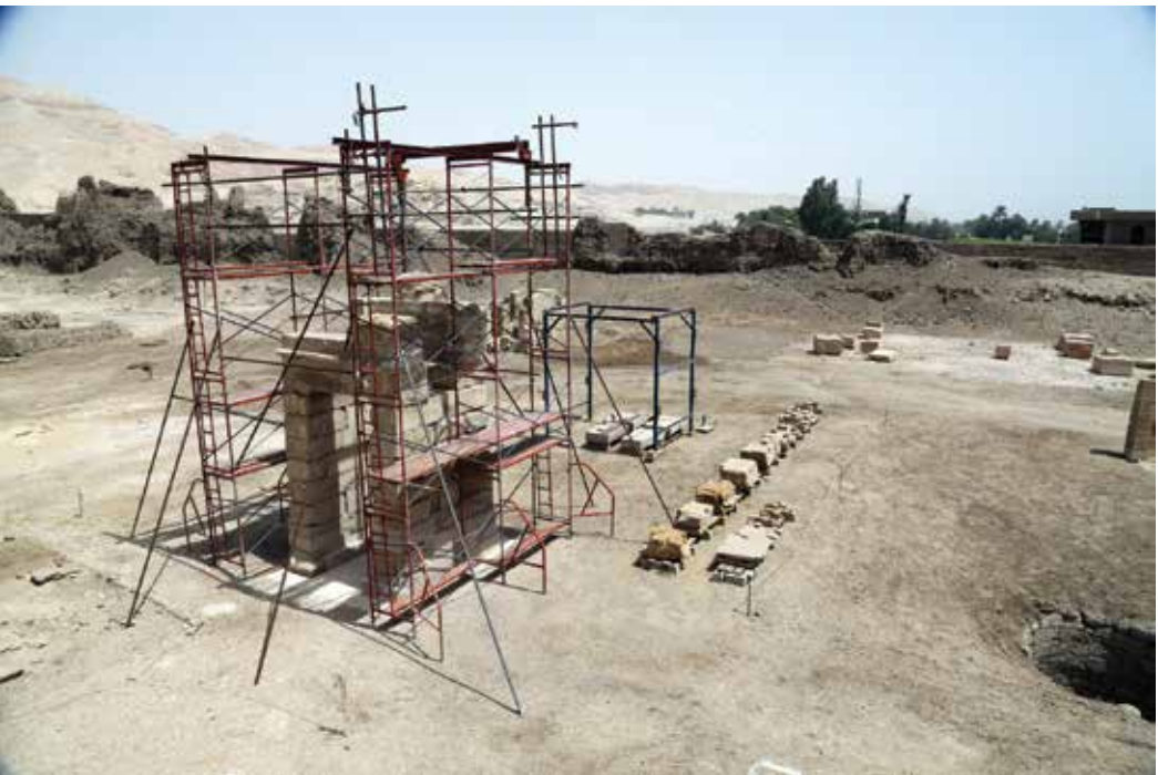
Figure 17. View of the Domitian Gate reconstruction in progress, Medinet Habu (photo: Frank Helmholz)
