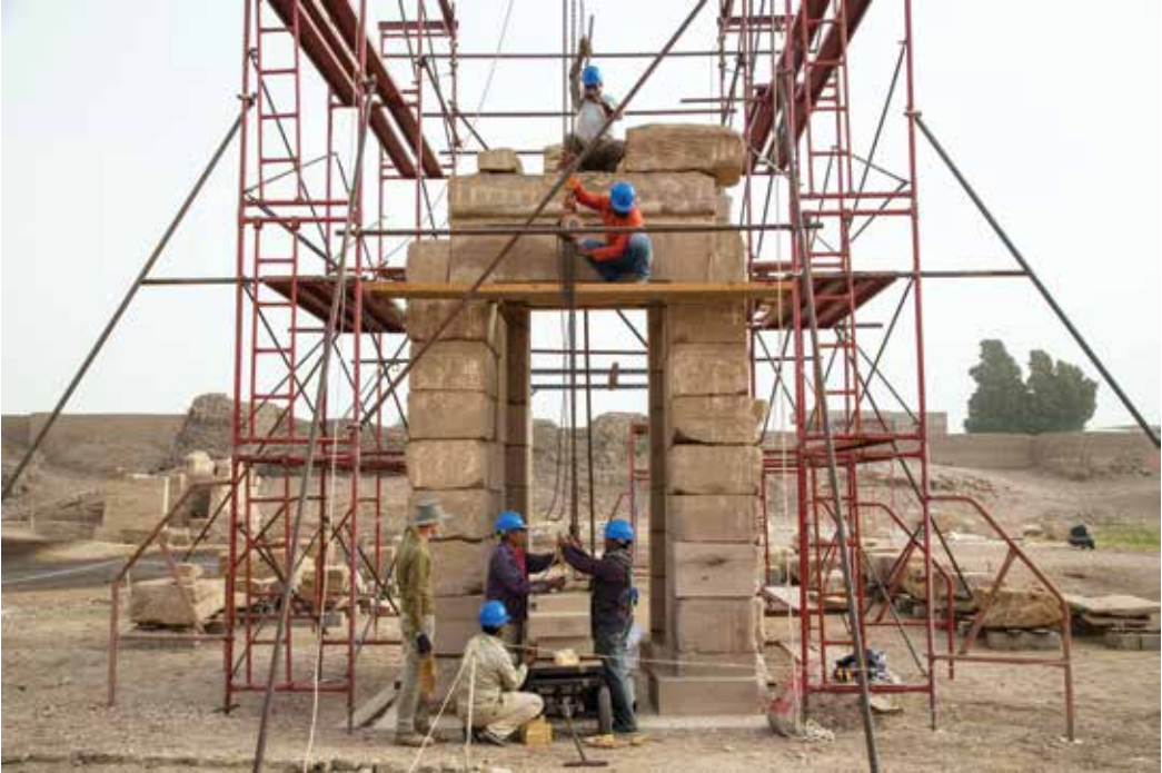
Figure 16. Johannes Weninger and Chicago House workmen reconstructing the Domitian Gate, Medinet Habu (photo: Ray Johnson)
