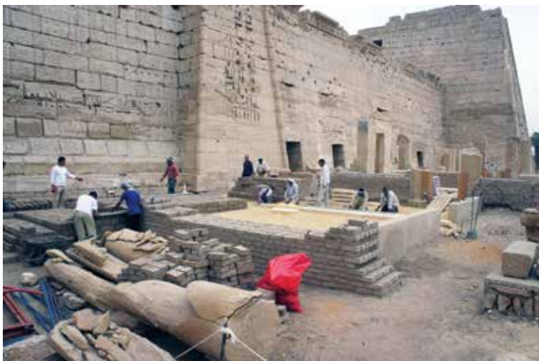
Figure 6. Construction of stone viewing platform with restored mudbrick walls. Ramesses III palace, Medinet Habu (photo: Ray Johnson)
