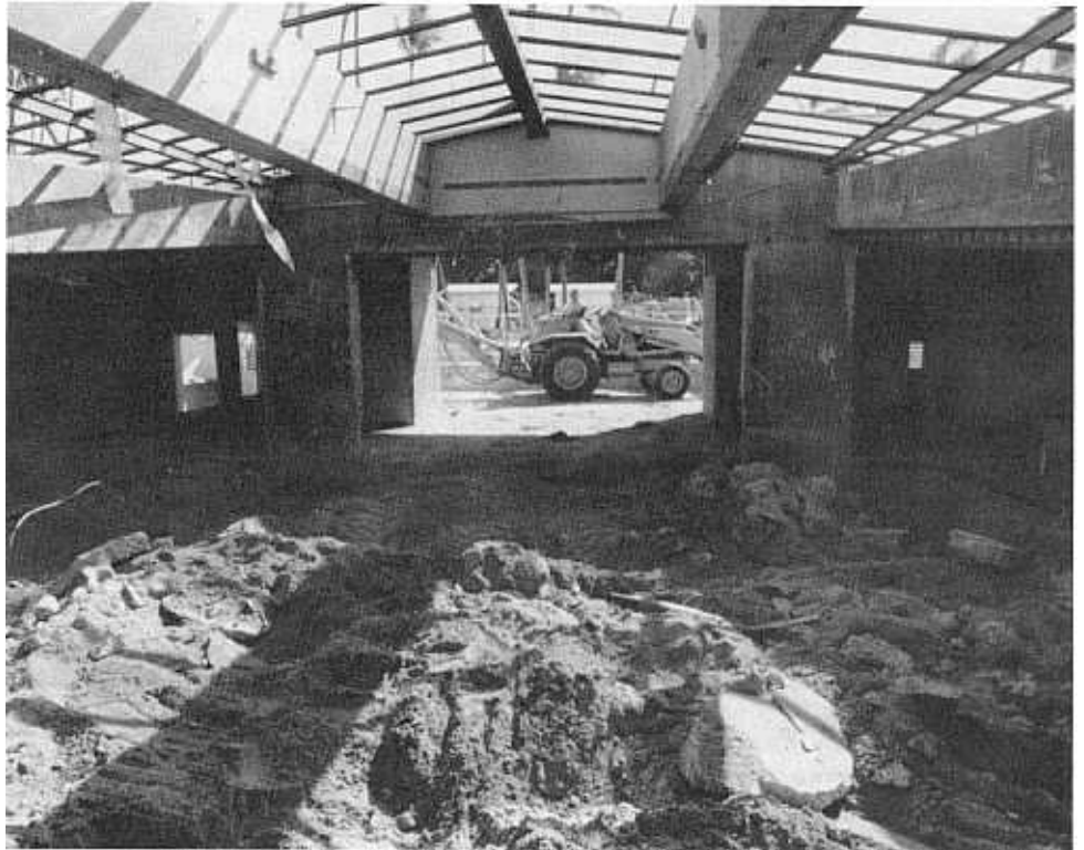
Tom Kelly photo courtesy Waikiki Aquarium Demolition of the Waikiki Aquarium's old shark tank has been completed; the new "Hunters of the Reef" display taking its place will be four times larger. The photo looks out from what used to be the behind-the-scenes staff work area. Construction of the new exhibit will be under way by mid-April.
