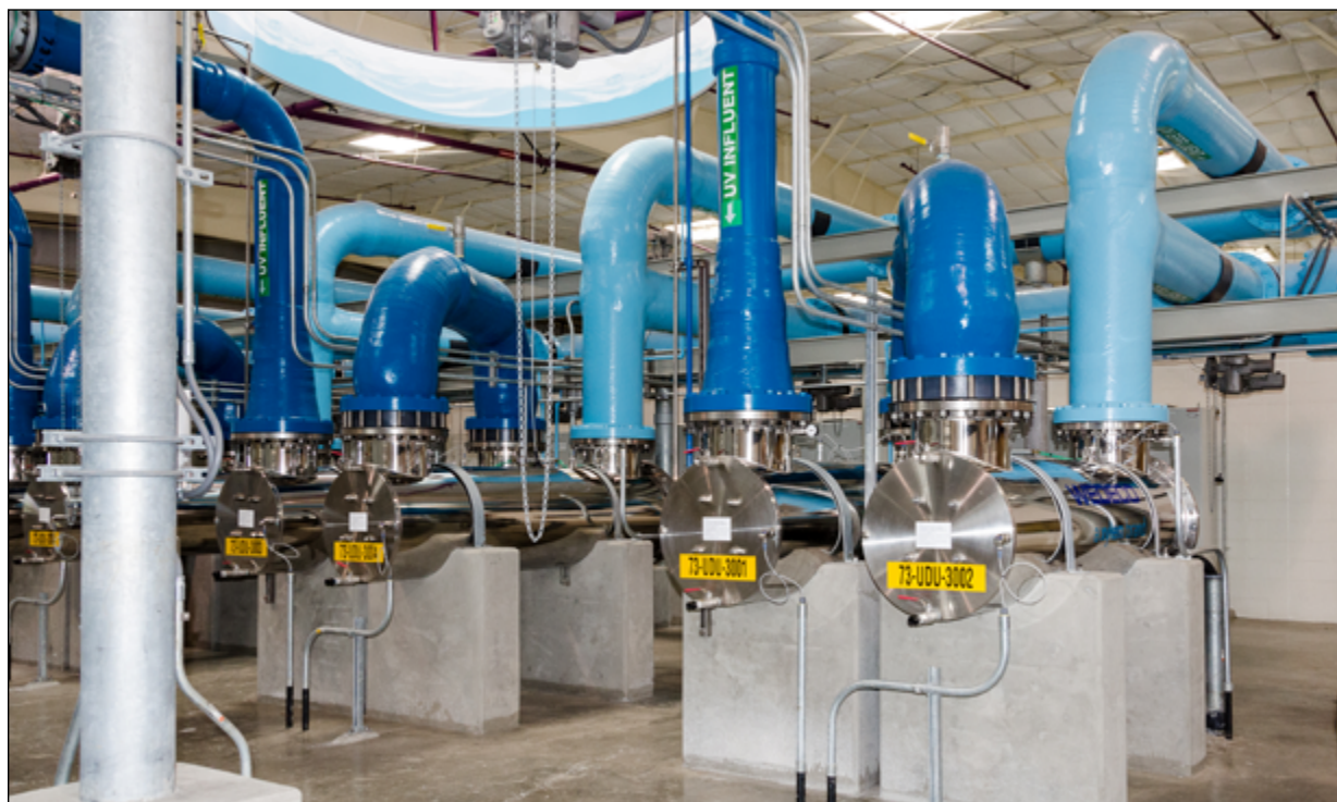
Prolonged drought and extreme heat may create more demand for recycled water that has undergone ultraviolet or other treatment in facilities like this one.
