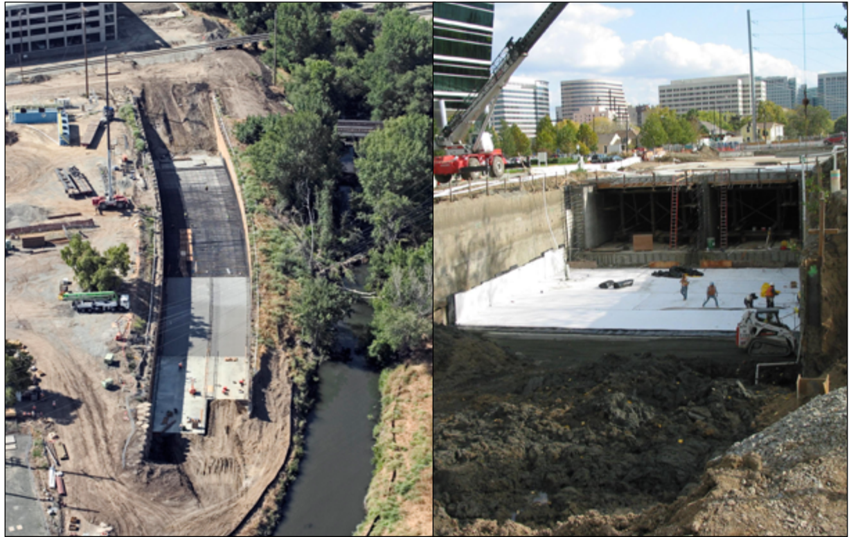
In an example of the natural flood protection approach, the District designed the Guadalupe River Project through downtown San Jose to protect more than 7,000 properties from a one percent risk of flooding, while also improving the river's ecology, hydrology, fisheries, and habitat. In partnership with the Corps, the District widened and planted extensively in the floodplain and upland areas to decrease erosion and increase habitat space. Upriver, the District is working to stabilize the channel and expand habitat for steelhead trout and other native fish. Photos: SCVWD
