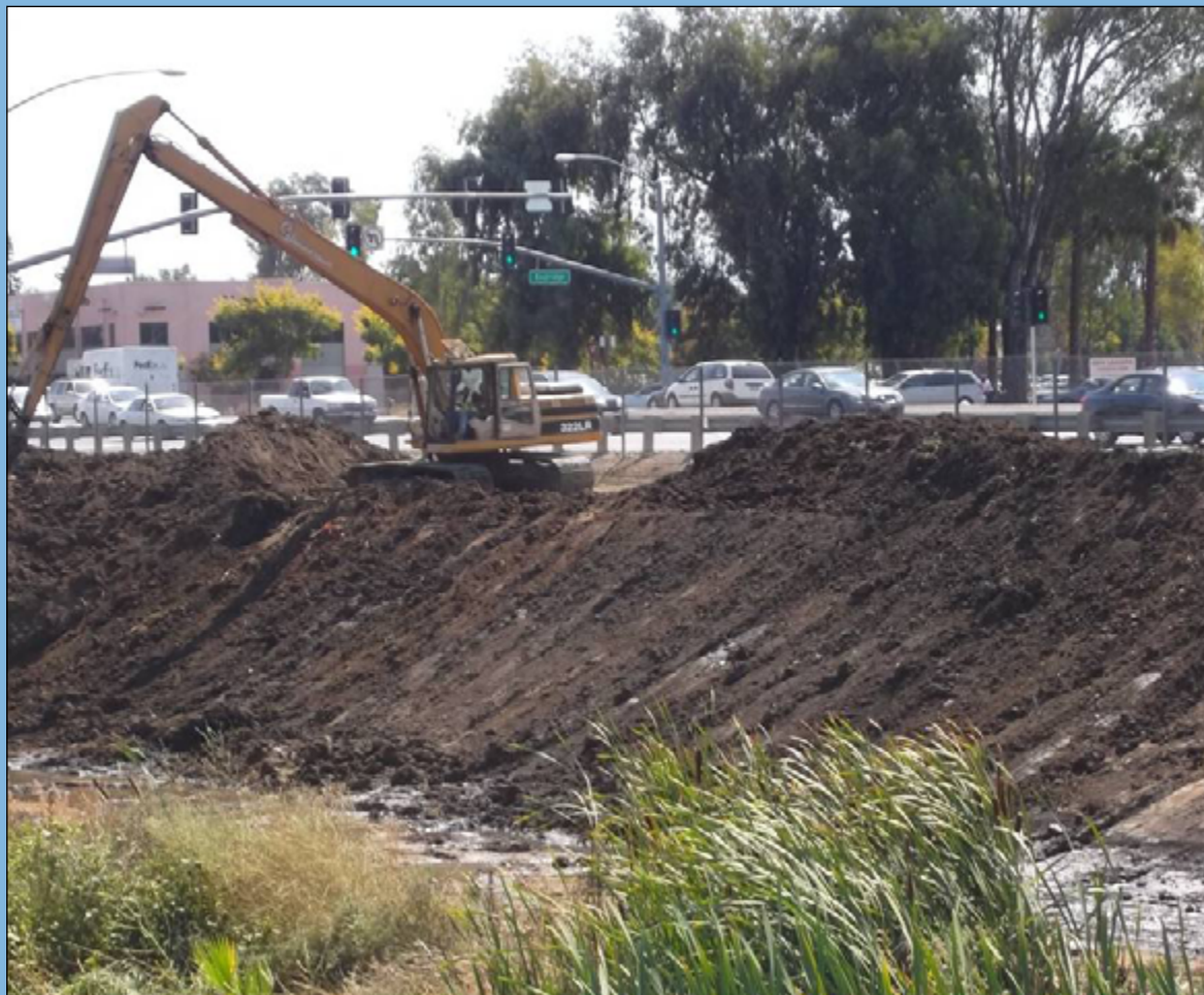
Removing sediment from Thompson Creek, San Jose, to maintain stream capacity and condition. Photo: SCVWD
