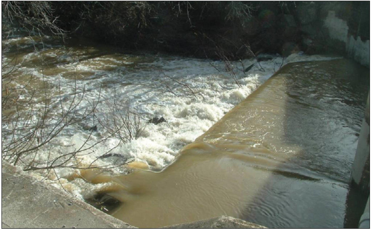
Bolsa fish ladder on Uvas Creek in the Pajaro River watershed at the Union Pacific Railroad crossing. Photo: Valley Water
