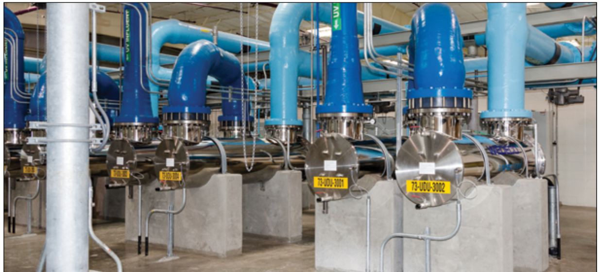
Prolonged drought and extreme heat may create more demand for recycled water that has undergone ultraviolet or other treatment in facilities like this one.
