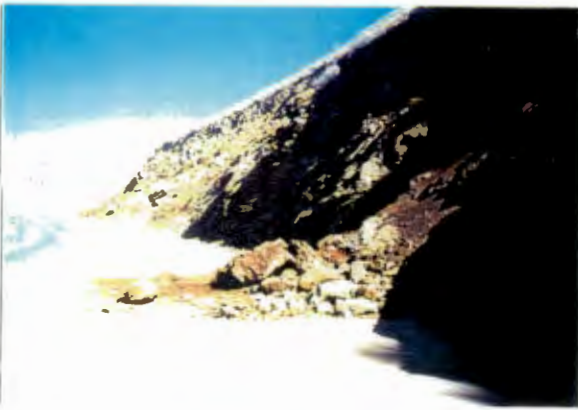
Plate 5.3a Soil creep along the slope of the northern access road.
