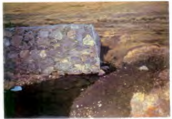
Plate 5.4d Eroded channel, around the gabions.
