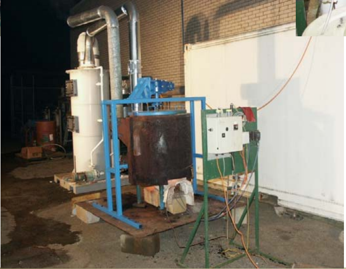
Mini pilot plant roaster and off-take gas scrubber
