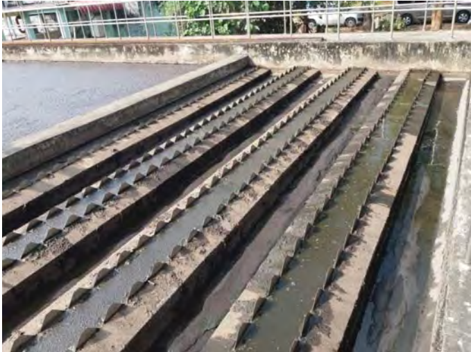
No.7 Primary Settling Tank (Overflow Trough)
