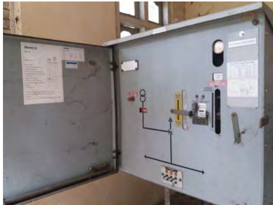
No.1 Incoming Panel
