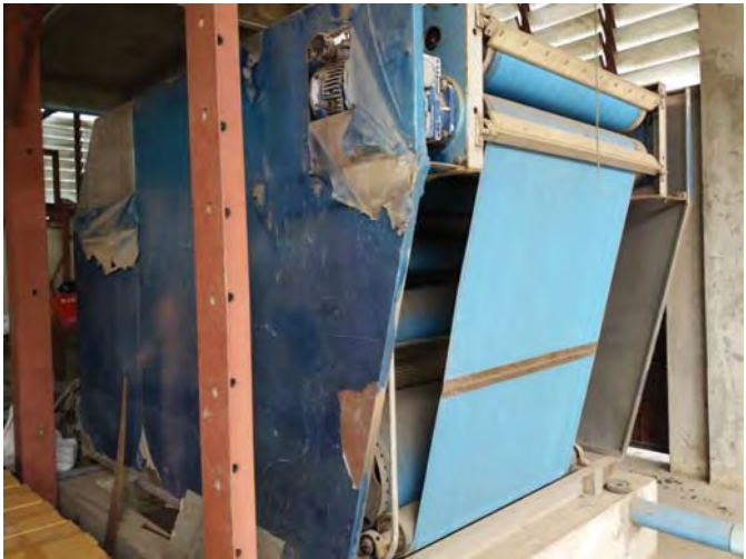
No. 13 Sludge Dewatering Unit (Belt Press 1mW)
