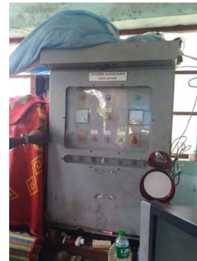
No.8 Return Sludge Pump Panel
