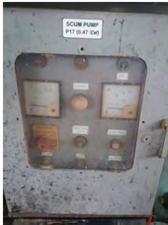
No.9 Scum Pump Panel
