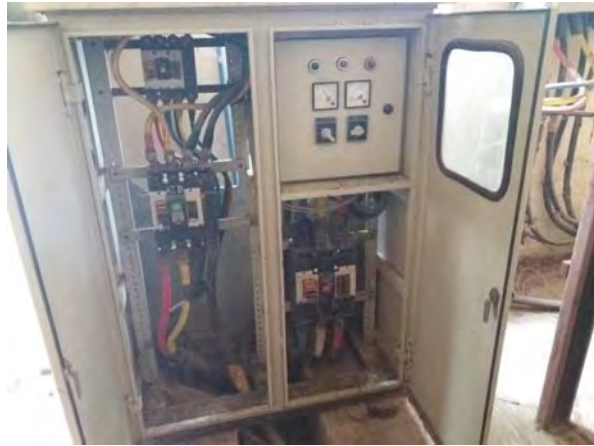
No.5 Distribution Panel (2)
