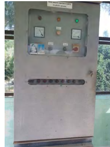
No.11 Raw Waste Water Pump Panel
