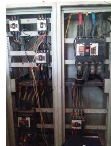
No.4 Distribution Panel (1)
