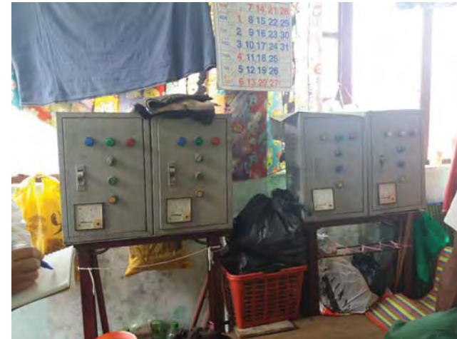
No.7 Secondary Settling Tank Scrapers & Thickener Scrapers
