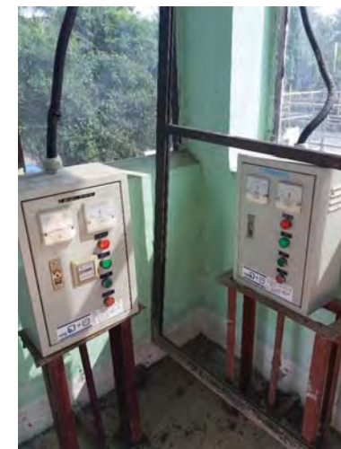
No.12 Grit Separator & Grit Pump
