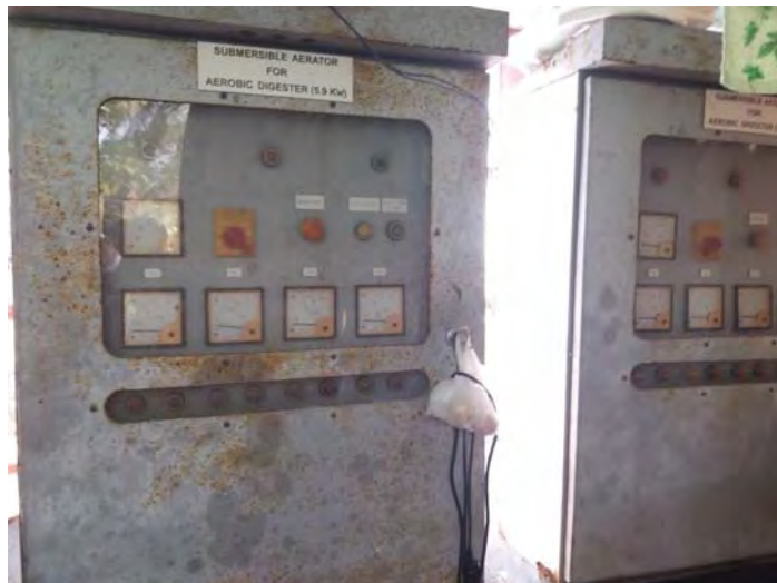
No.6 Aerobic Digester Control Panel
