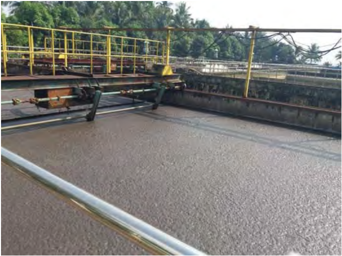
No.6 Primary Settling Tank (Scraper)
