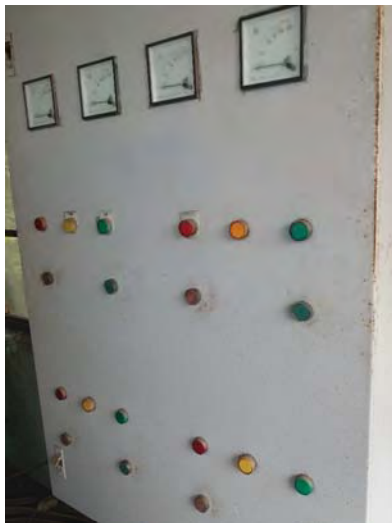
No.10 Surface Aerator Panel
