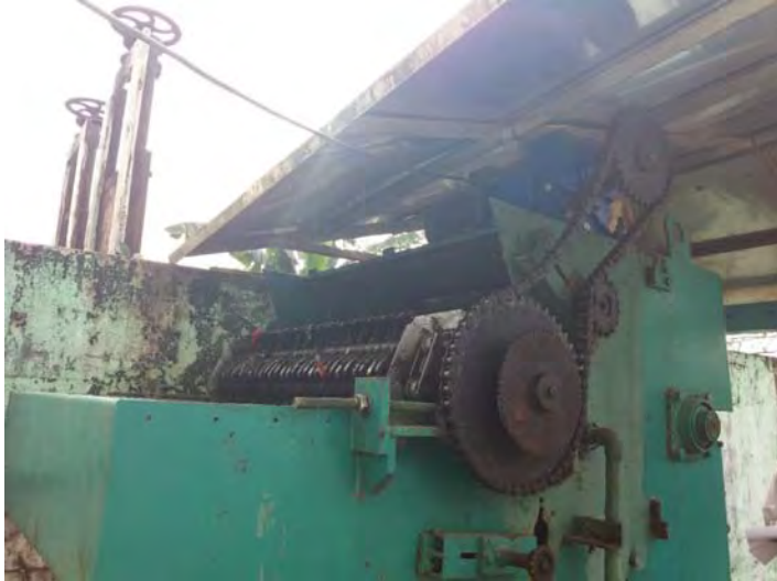
No.3 Auto Bar Screen (Drive Side)
