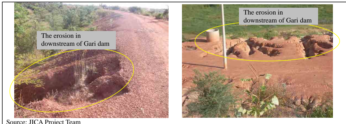
Photo-2 Erosion Status in Gari Dam Body
