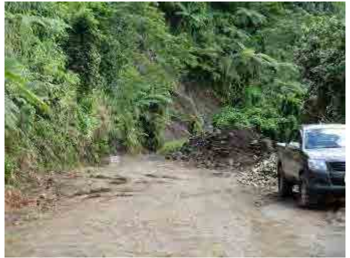
Photo-2 Condition of landslide along approach road to weir
