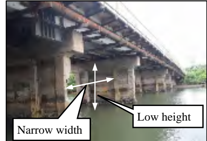
Photo 2-2-6 Current bridge has a narrow width and low height
