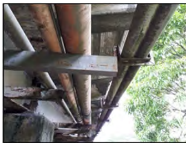
High voltage electric power lines and communication tubes
