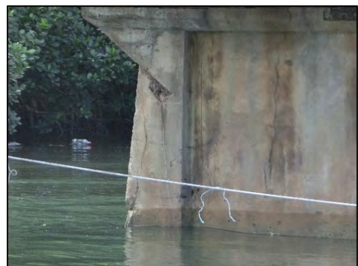
Photo 2-2-5 Concrete cracks in bridge piers (Bridge B)
