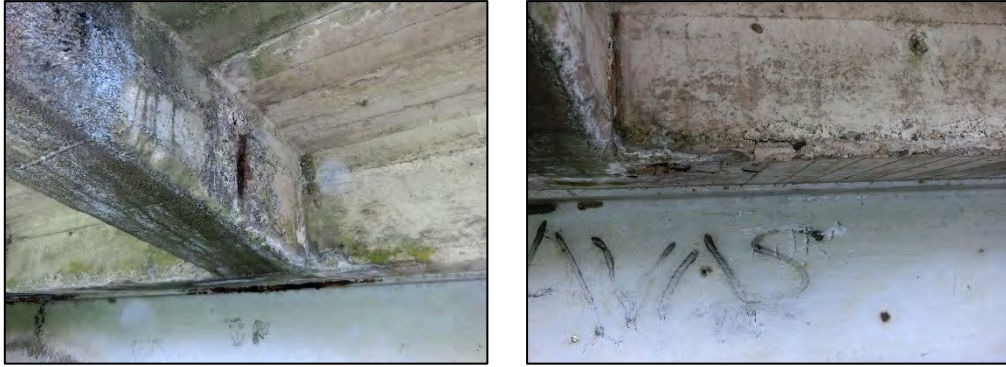
Photo 2-2-3 Areas with poor construction work including honeycombs and construction joints and areas with insufficient covering
