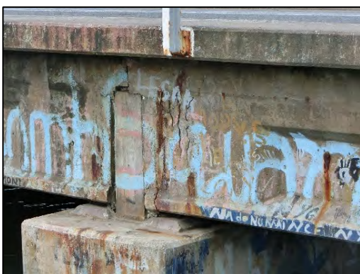
Photo 2-2-4 Concrete flaking from rebar corrosion (Bridge A)
