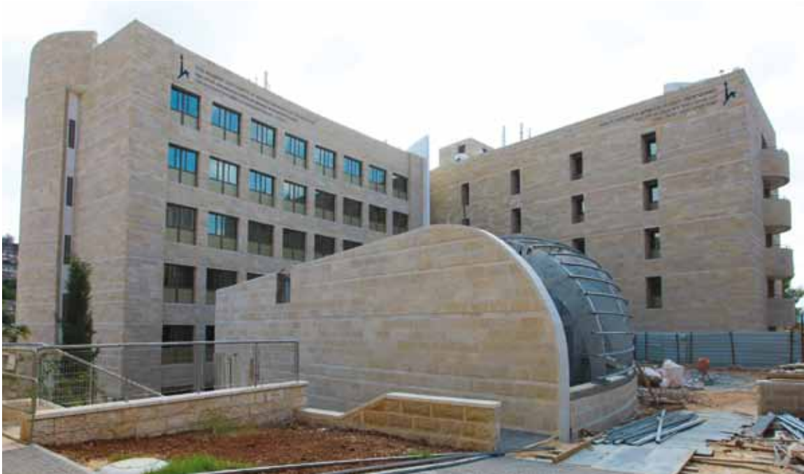
Construction of the Octav and Marcela Botnar Medical Research Building, Ein Kerem campus
